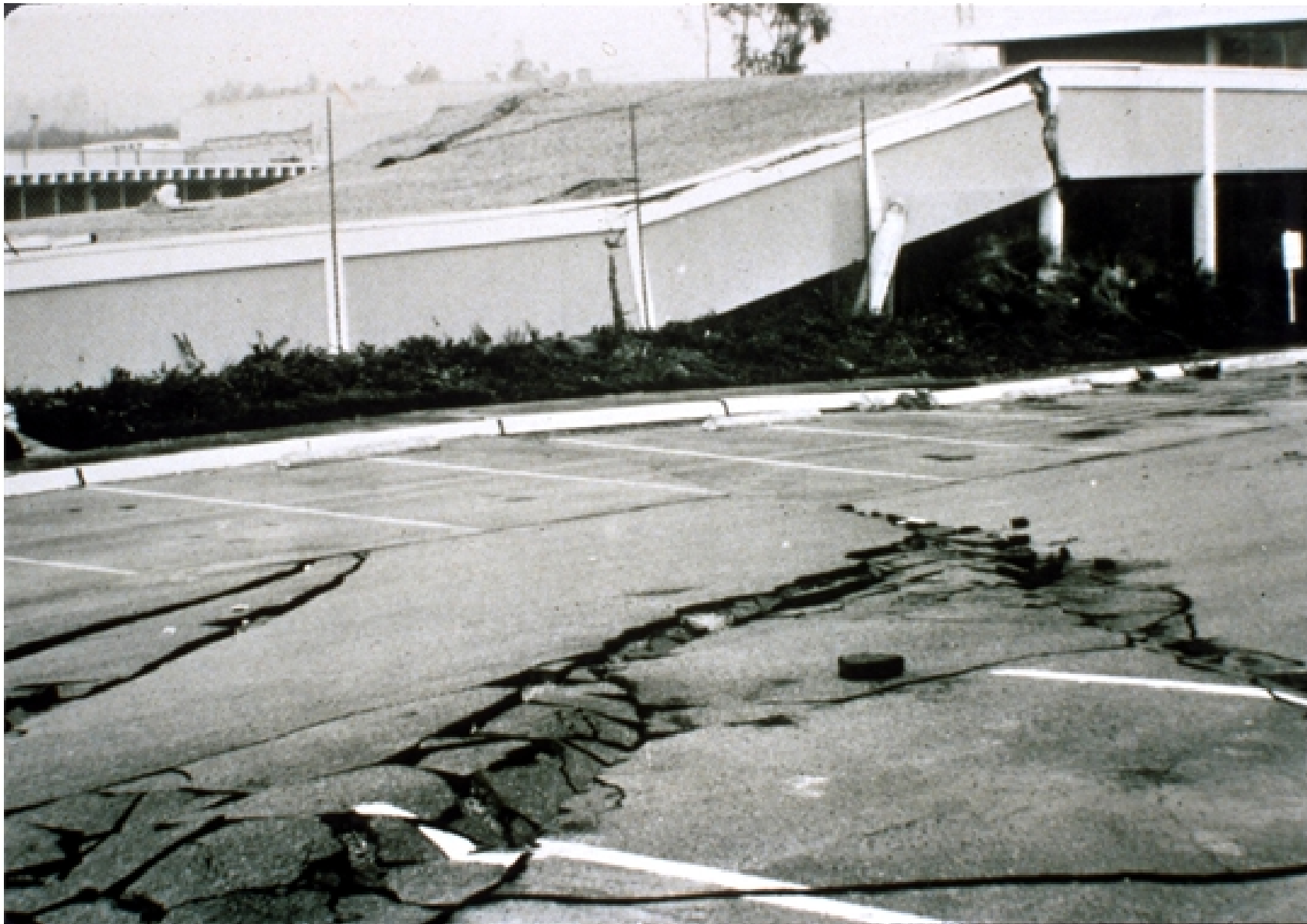
Fig. S5. Collapsed court building at SFJH; collapse caused by differential shear displacement beneath the building; right end of the building displaced about 0.9 m toward the camera relative to the left end which remained nearly in place (T.L. Youd photo)
