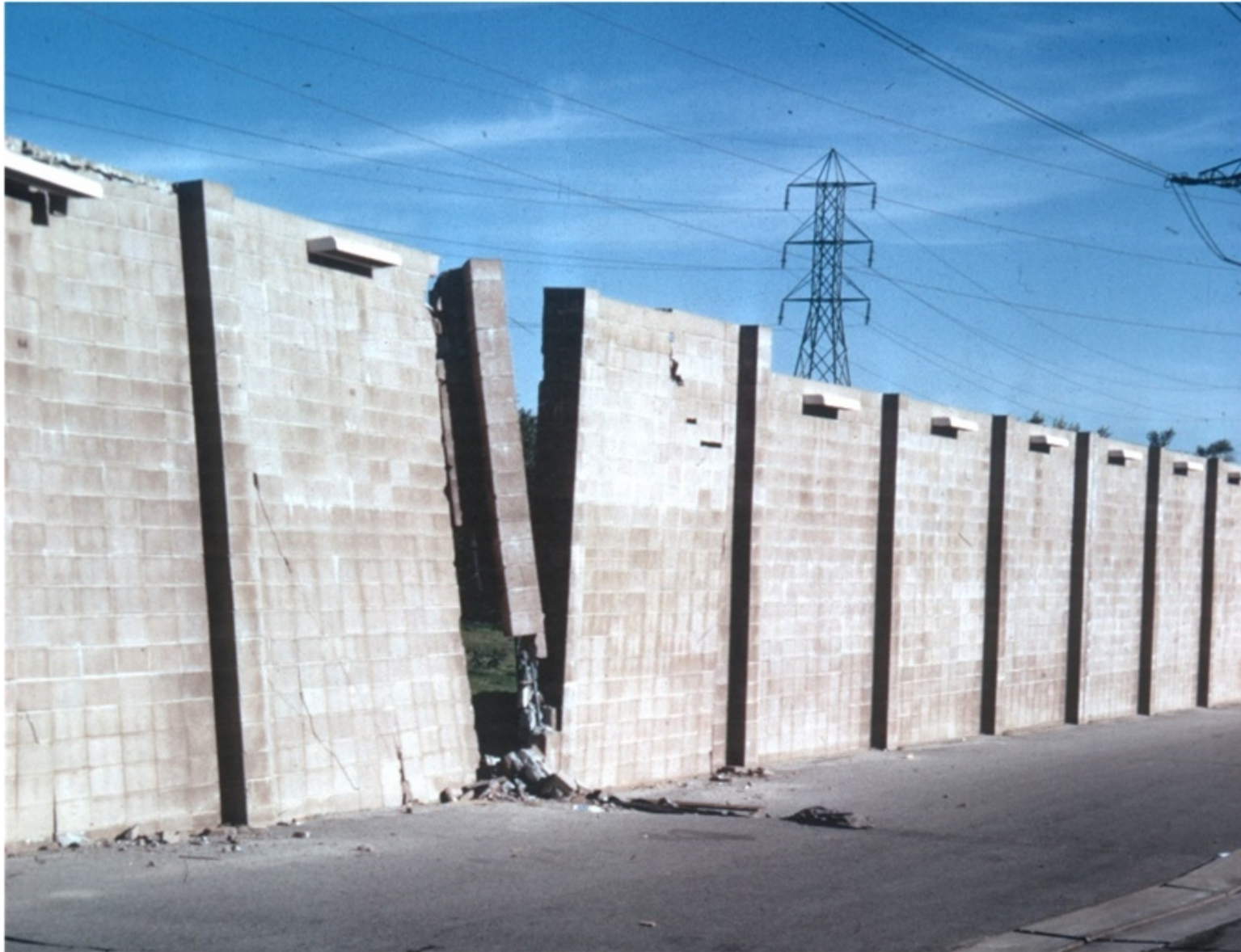
Fig. S7. Wall at JFSH pulled apart by lateral spread movement; about 50 juvenile inmates escaped through the fractured wall immediately after the earthquake (T.L. Youd photo)
