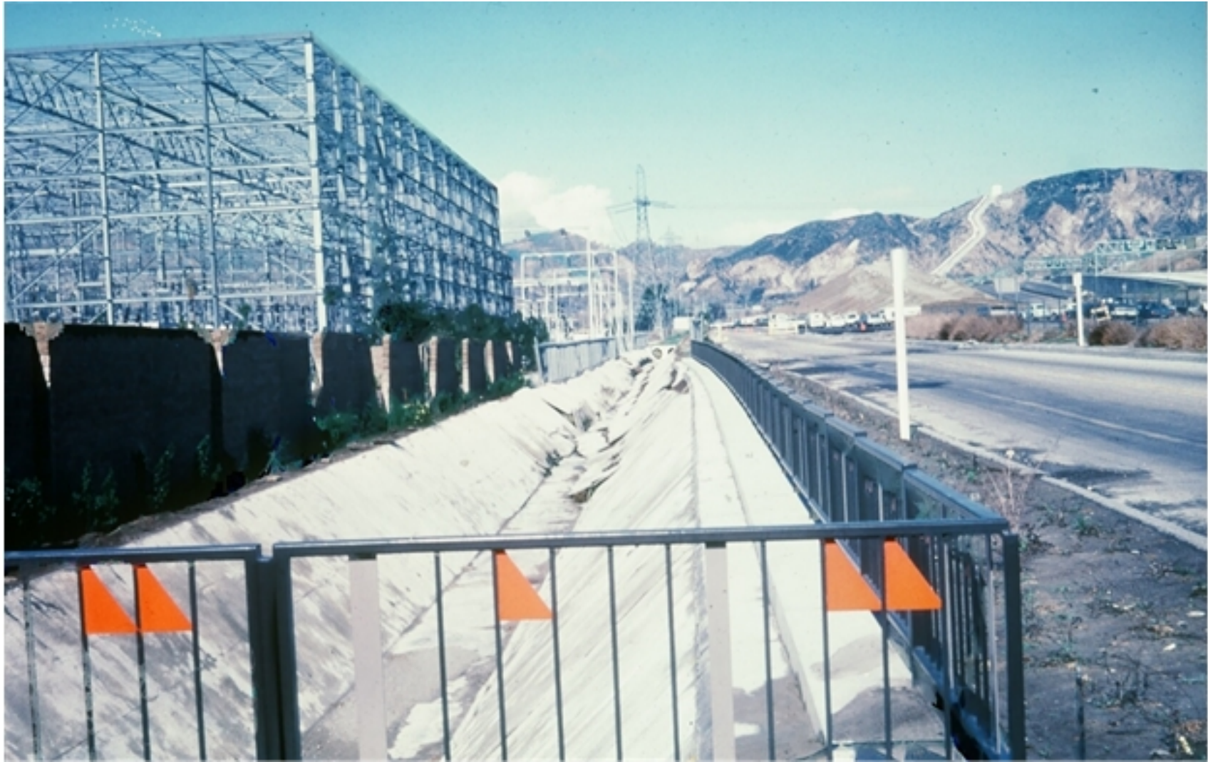
Fig. S3. Flood control channel compressed by SFJH lateral spread; channel acted as a partial toe for the spread (T.L. Youd photo)
